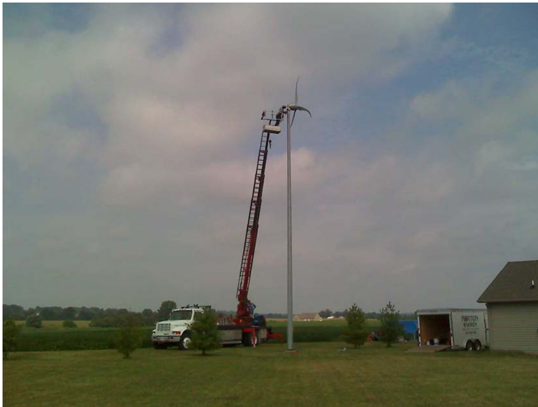
Skystream 3.7 Wind Turbine on 45' tower located in Warrenton, Indiana.
