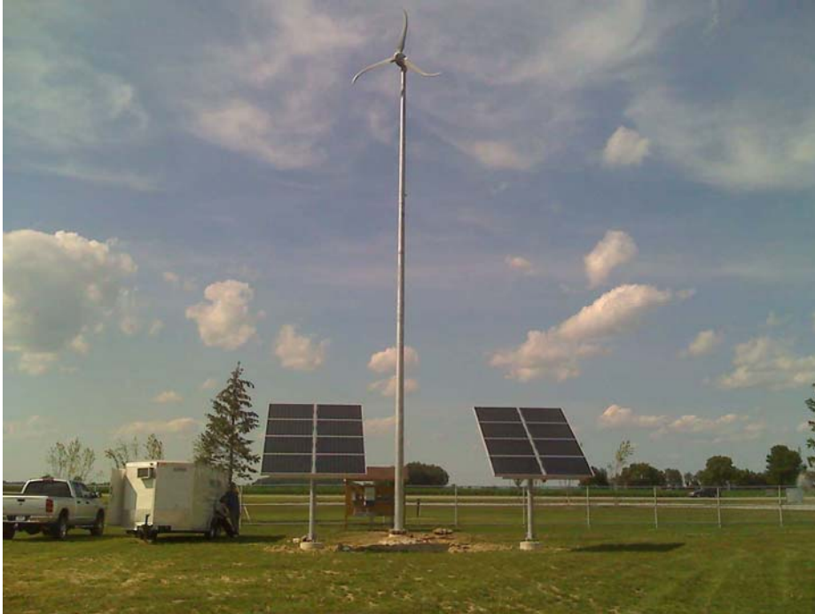
Wind/Solar Hybrid System 3KW Solar & Skystream installation at RushShelby Energy in Manilla, Indiana. Comp. in July 2009 (16) Sanyo Bifacial Solar Modules Owner: RushShelby Energy Coop, 2777 S. 840 W., P.O. Box 55, Manilla, IN 46150
