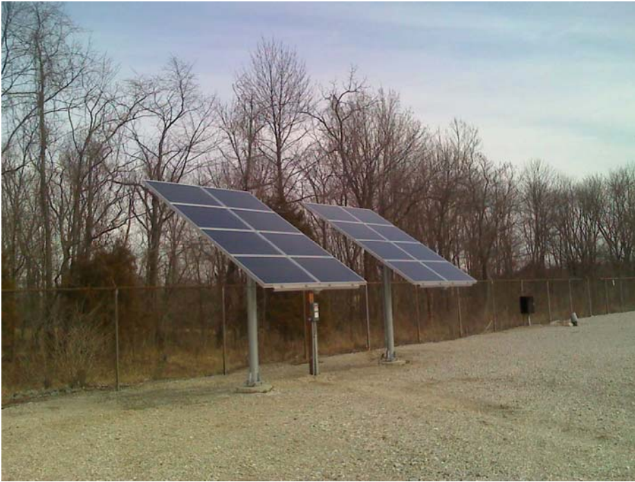
3KW Grid-Tied Solar installation at Hoosier Energy REC's Franklin Training Center in Franklin, Indiana
