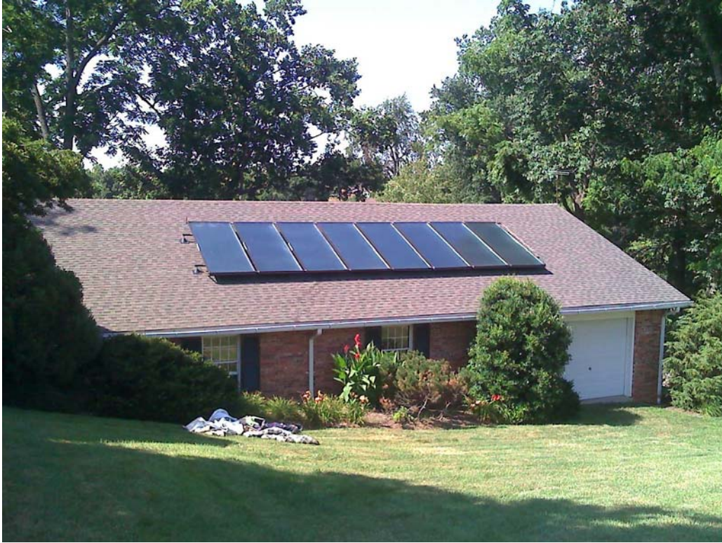
Solar Thermal Pool Heating System for Indoor Pool. Located in Newburgh, Indiana. Owner: Becky Edwards
