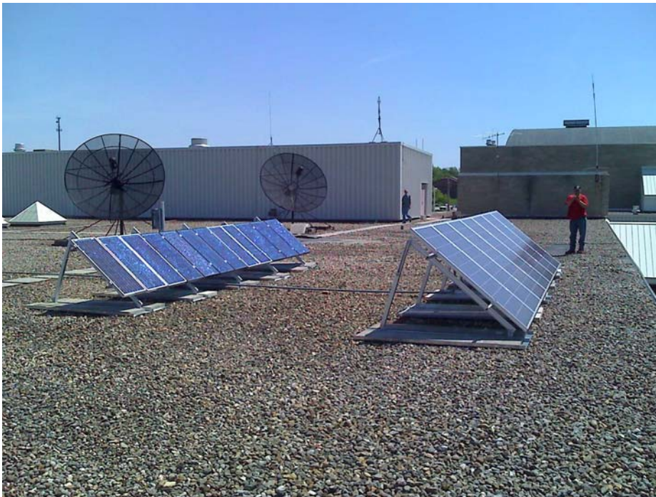
2.3KW Solar System at Bloomington South High School 1965 S. Walnut St. Bloomington, Indiana Owner: Cindy Kvale (812)330-7714
